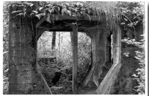
Press foundation at the brick factory.
