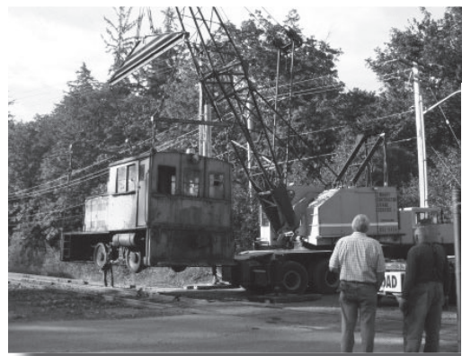
Above, Lifting the train off the tracks and onto a flatbed truck. Center - The Before picture right after it arrived, Pictured are Coke Roberts, Keith Watson and Howard Botts. Top right, Train after restoration!
