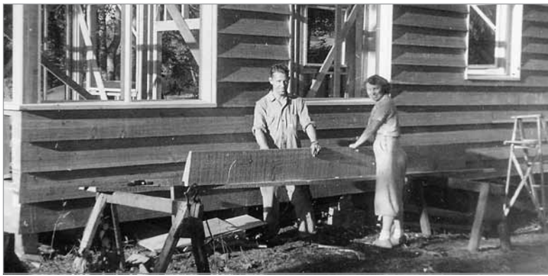
Under construction: The siding for the cabin was sawn at a mill at Henry's Switch, near where the Millwork Outlet is located today on SR 169. The siding is a "raked" cedar and almost impossible to replace, says Jack.
