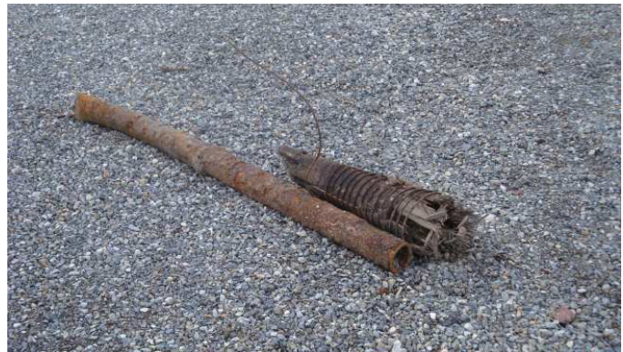
Some of the old water pipes were uncovered. All kinds of things were found under the old street.
