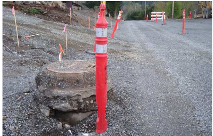
A man hole high and dry Portions of the street were lowered and some were raised.
